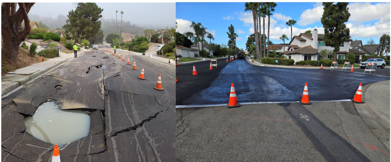
The site of the initial leak the morning of August 19 th (left), and the corner of Azahar St. and Cadencia St. after repaving (right).
