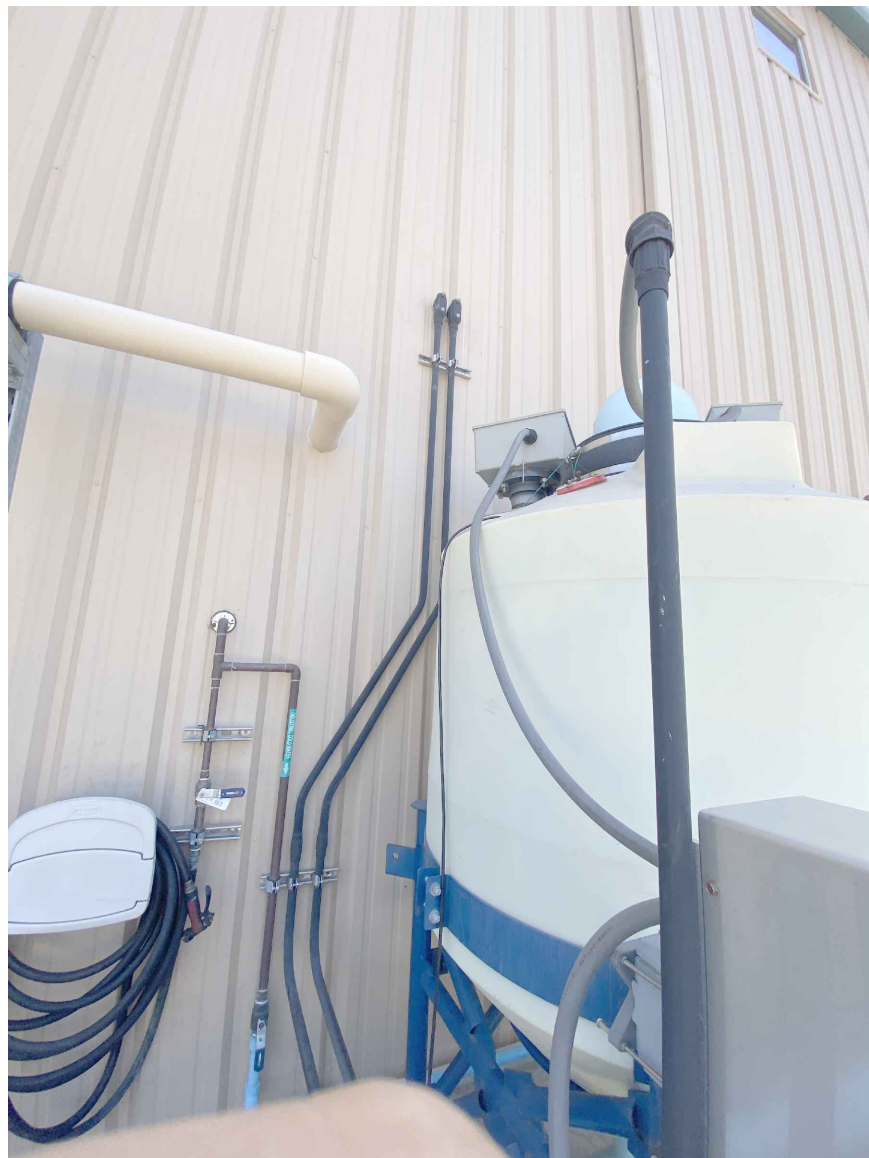
EXISTING CENTRATE TANK
