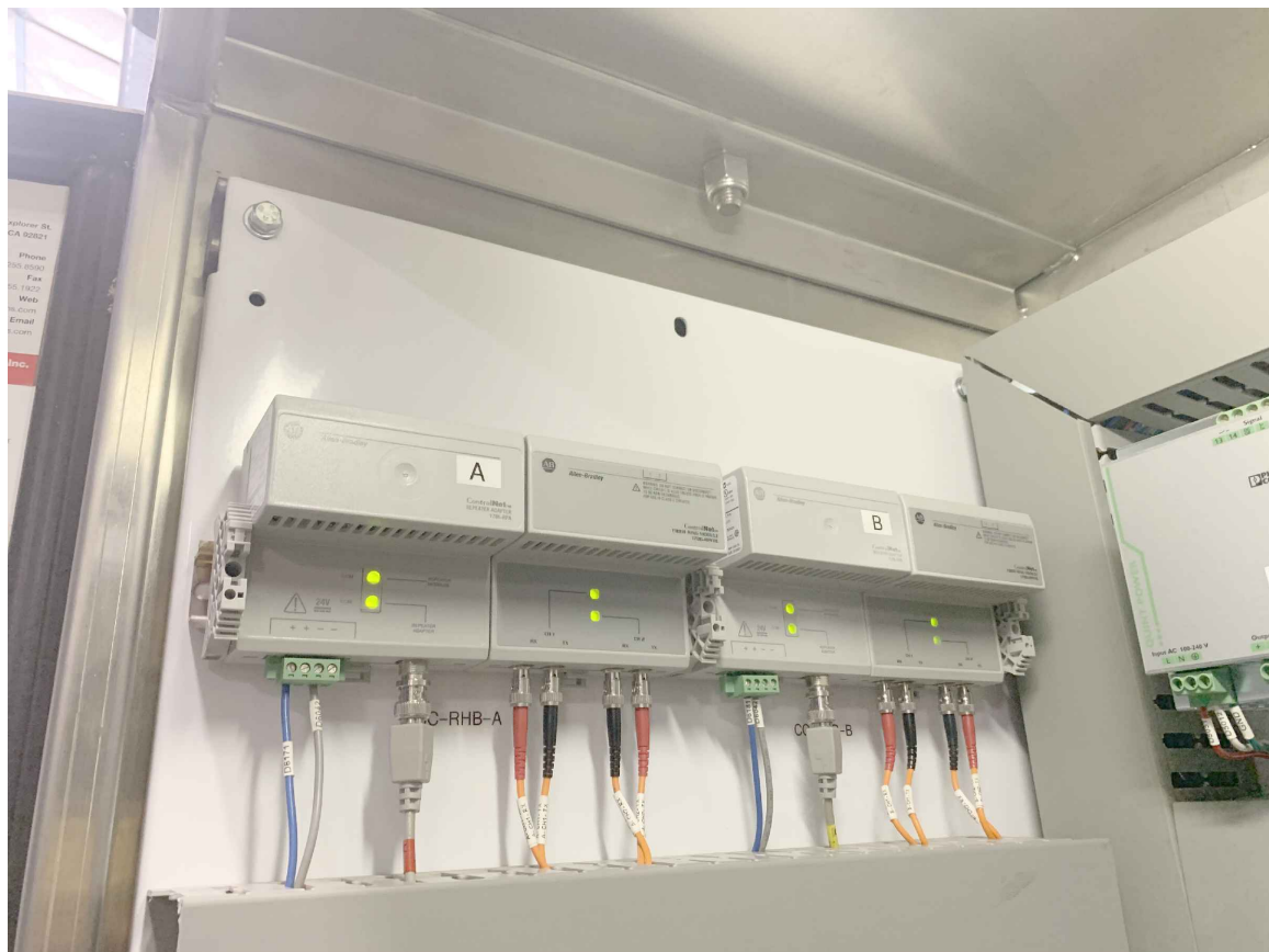
EXISTING PANEL CC-RHB LEFT SIDE PANEL NETWORK INTERFACE MODULES
