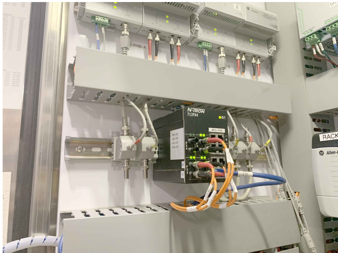
EXISTING PANEL CC-RHB LEFT SIDE PANEL NETWORK SWITCH
