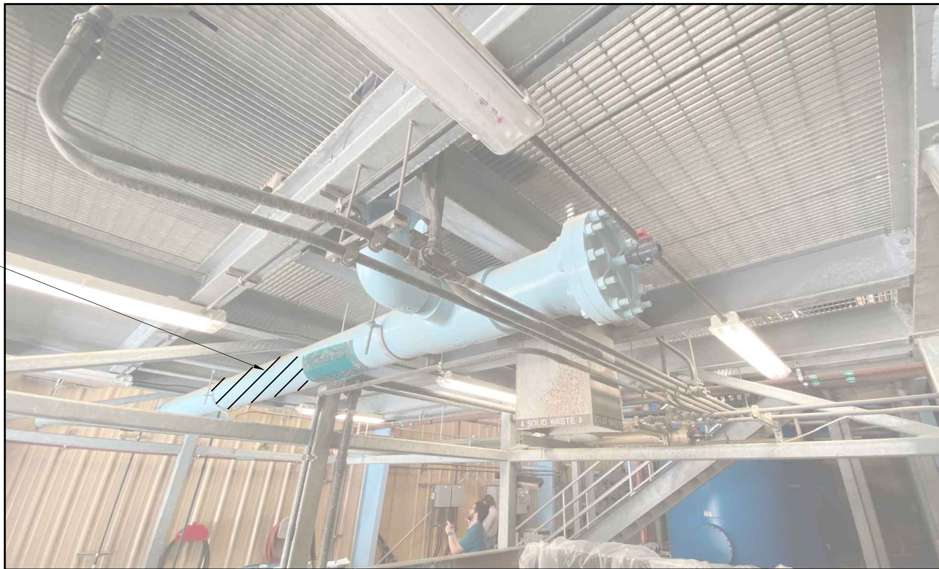
2 CENTRATE PIPING D-1
