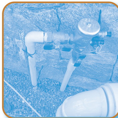
Backflow prevention device
