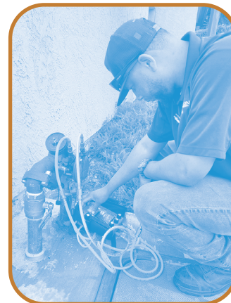
Backflow and Cross-Connection Coordinator Tim uses specialized equipment to test backflow device effectiveness.
