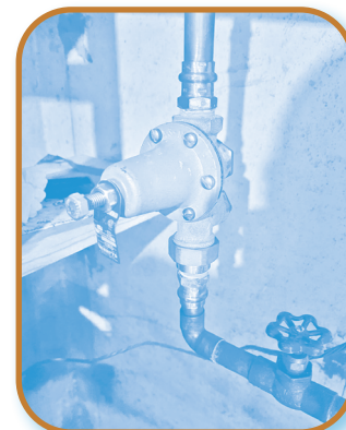
Pressure regulating devices are often located in a garage.
