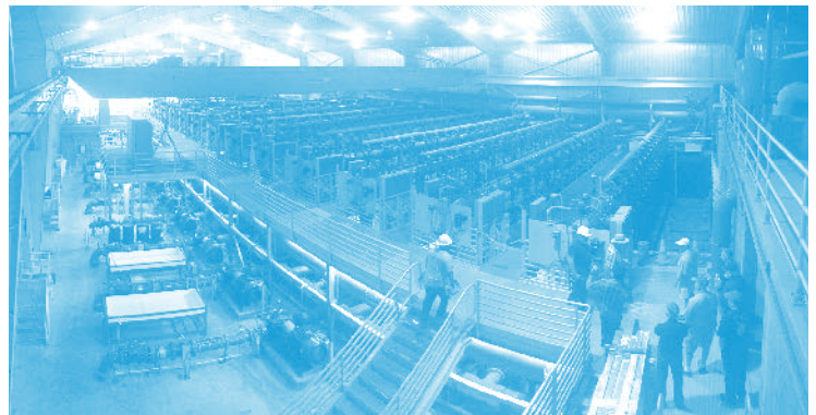
OMWD's David C. McCollom Water Treatment Plant
