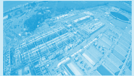
The Carlsbad Desalination Project is expected to produce drinking water in fall 2015
